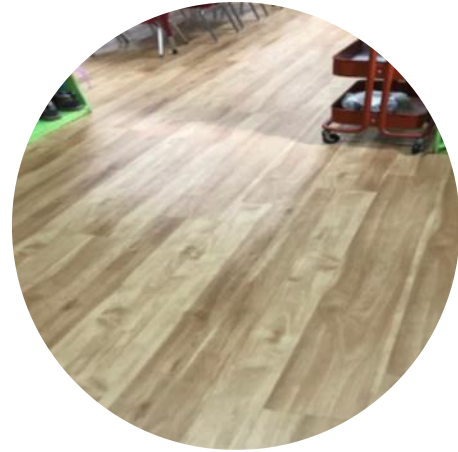
Damaged floor replaced. Courtesy New Jersey Economic Development Authority
